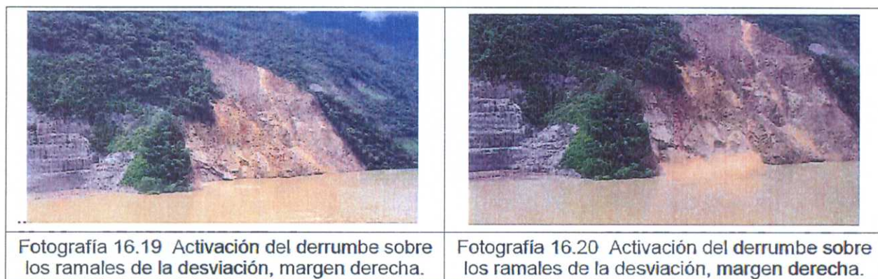
Figure 49. Reactivation of landslide above the Diversion tunnel intakes May 21, 2018 237
